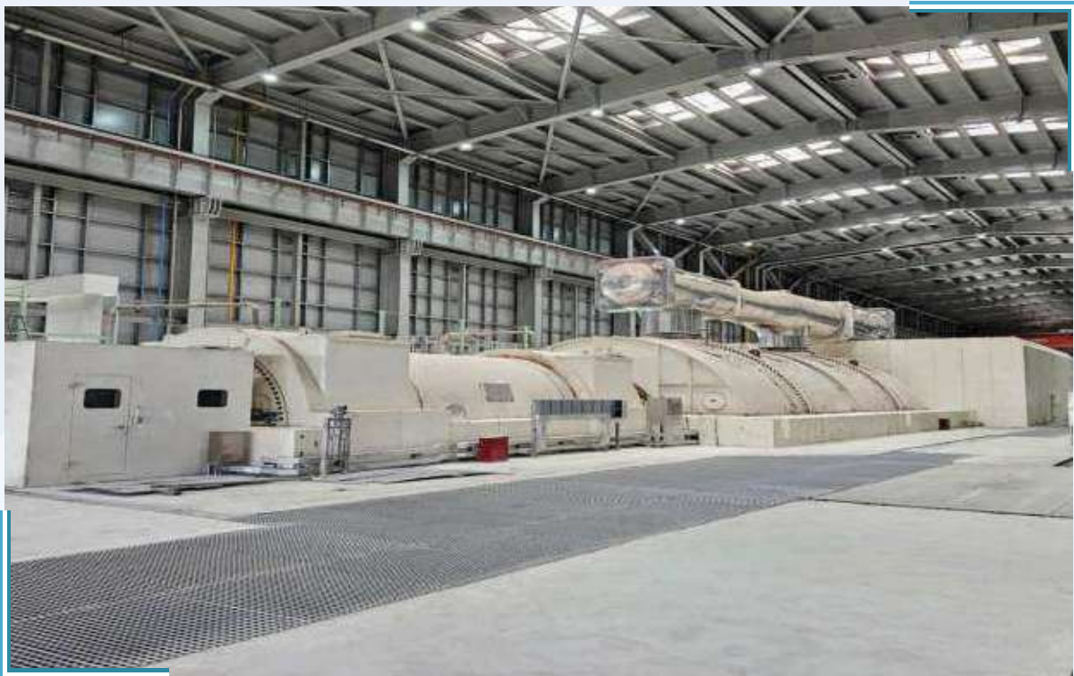
Turbine Generator (Unit 2)
