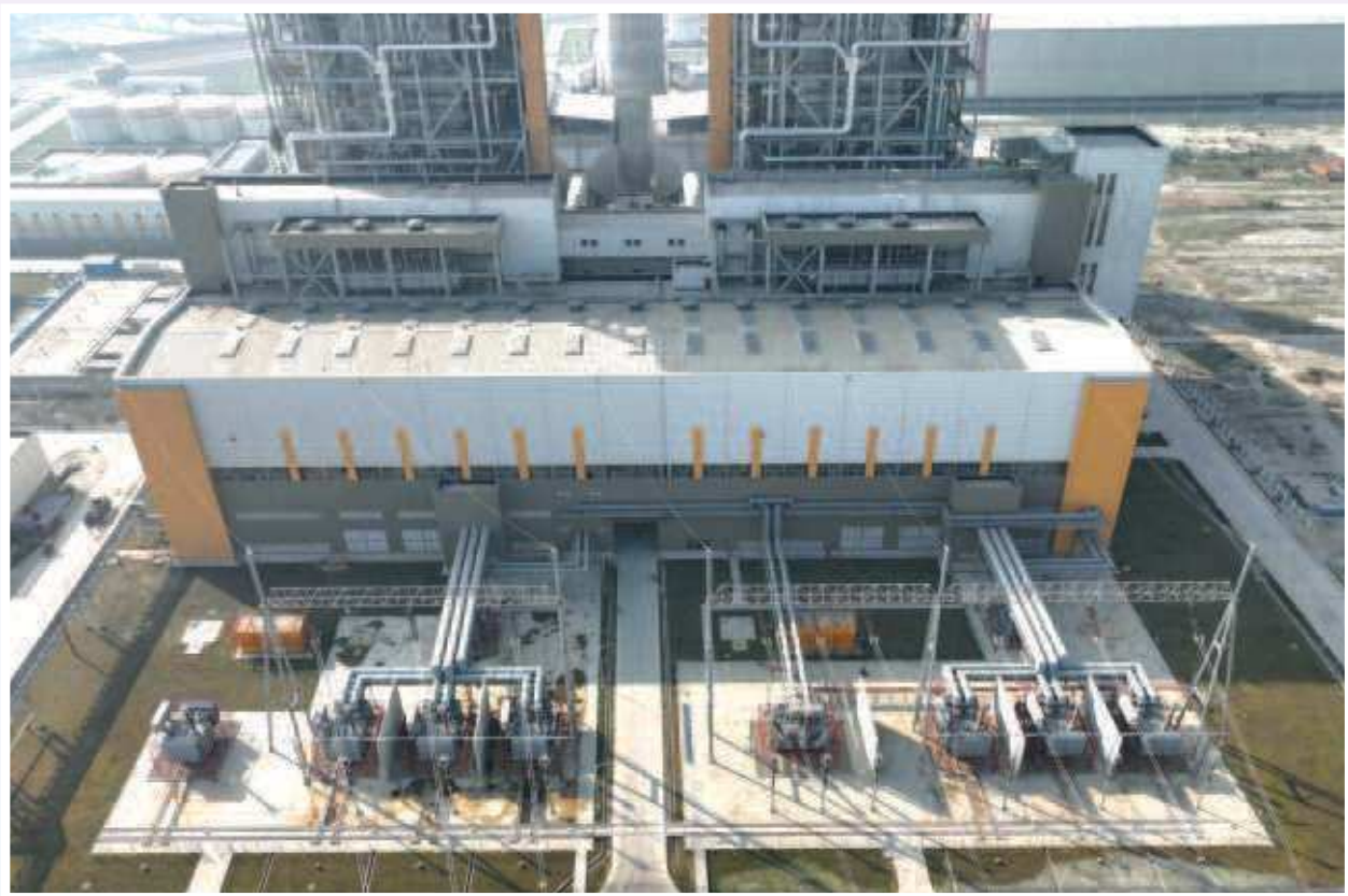
Generator Step Up Transformer
