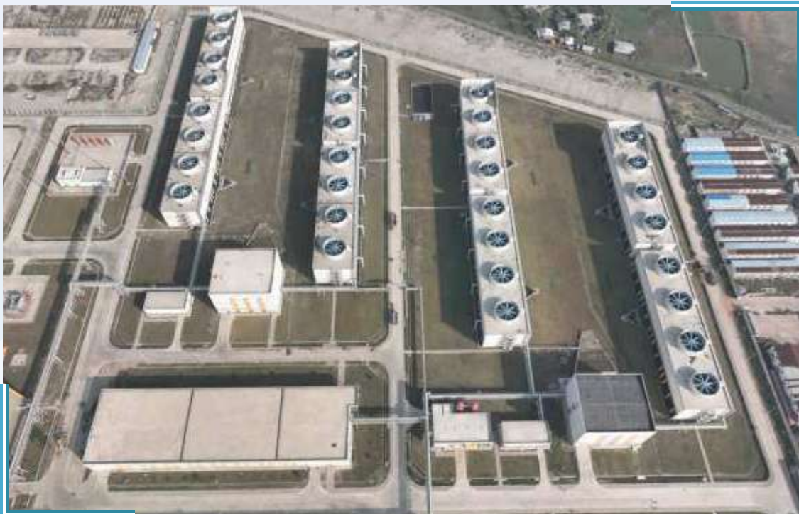
Cooling Tower Area
