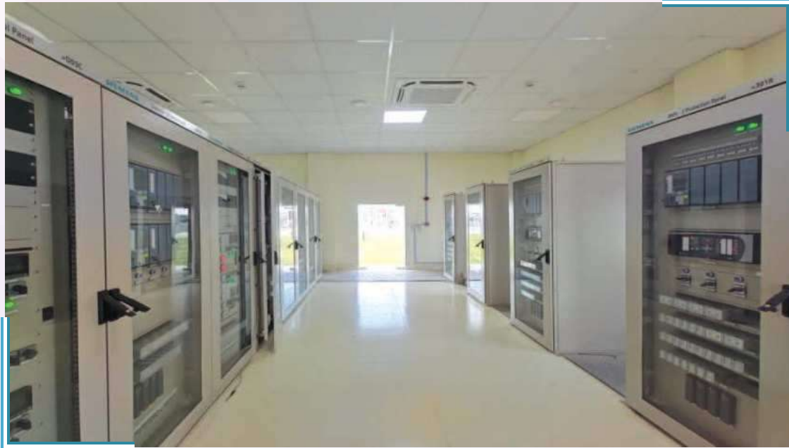
Amtoli 400 kV Switching Station Control Room
