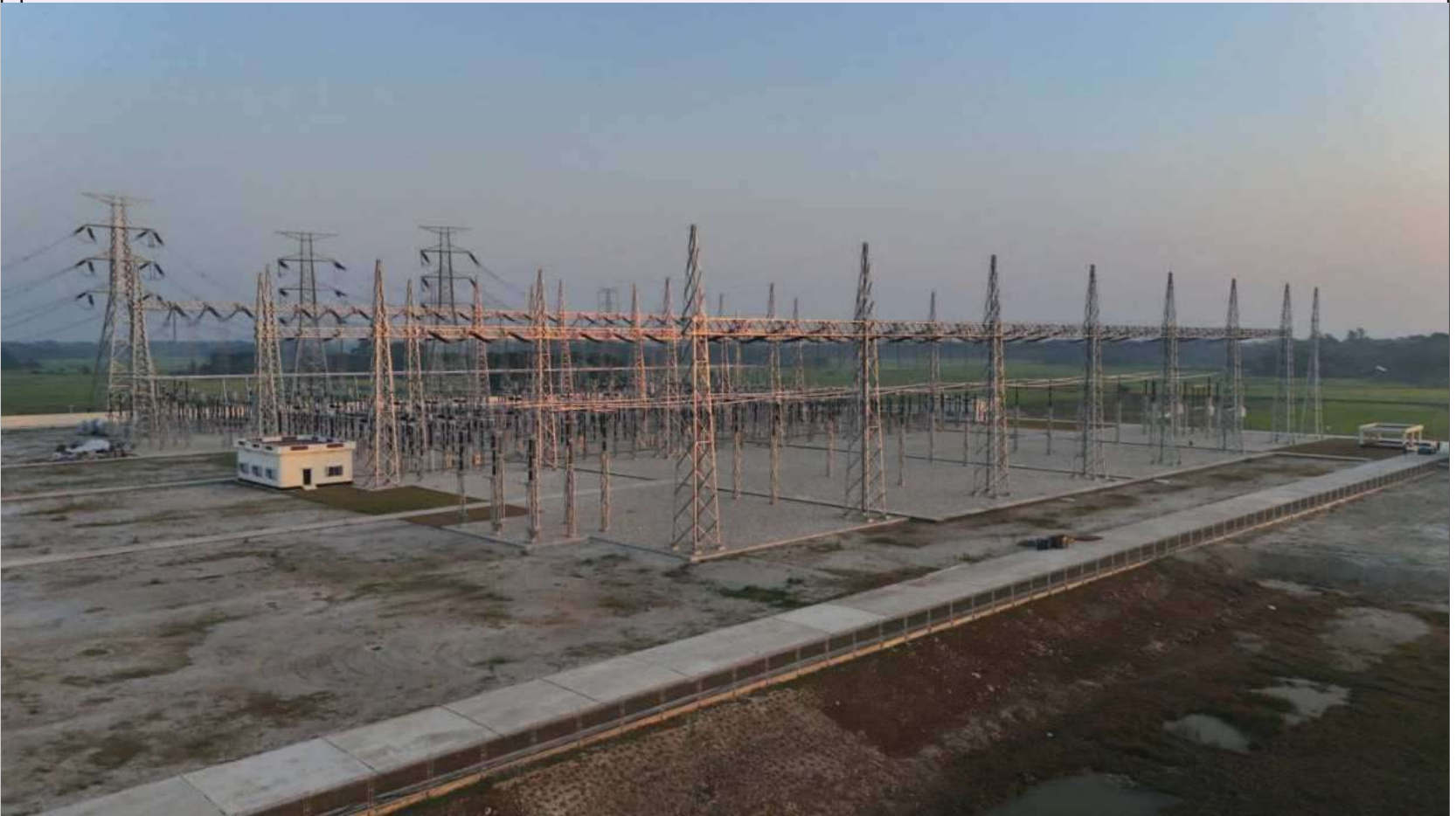
Amtoli 400 KV Switching Station
