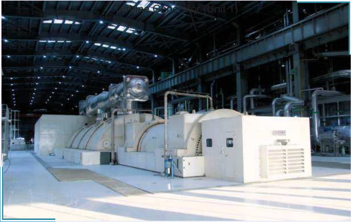
Turbine Generator (Unit 1)
